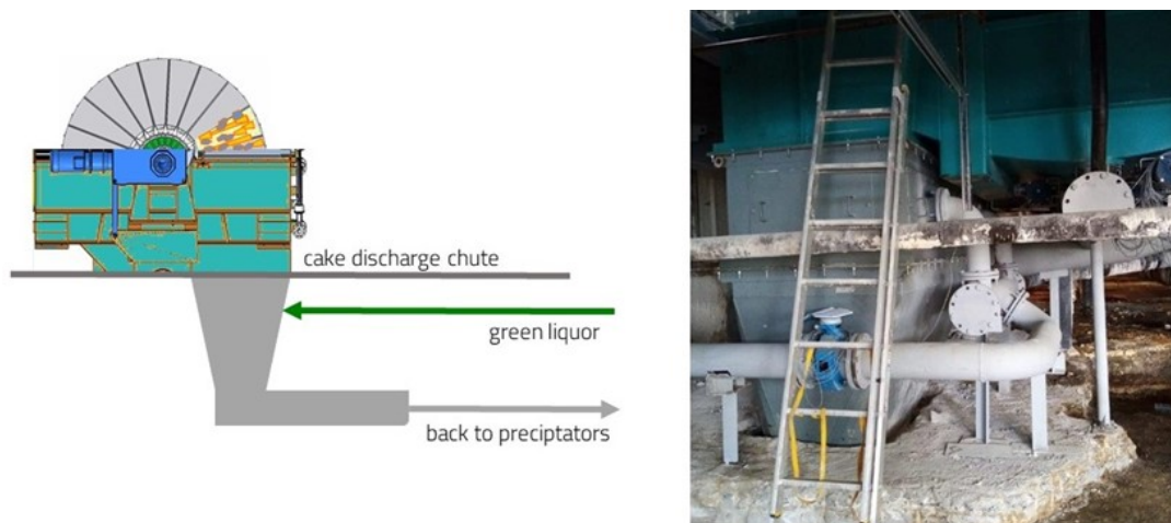
Figure 4. Disc filter with chute extension to allow for solids re-slurry.
